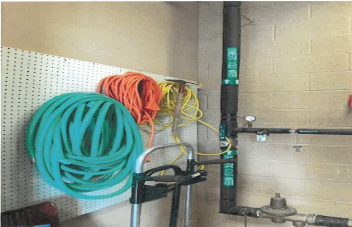
Utility room in Pool hallway.
