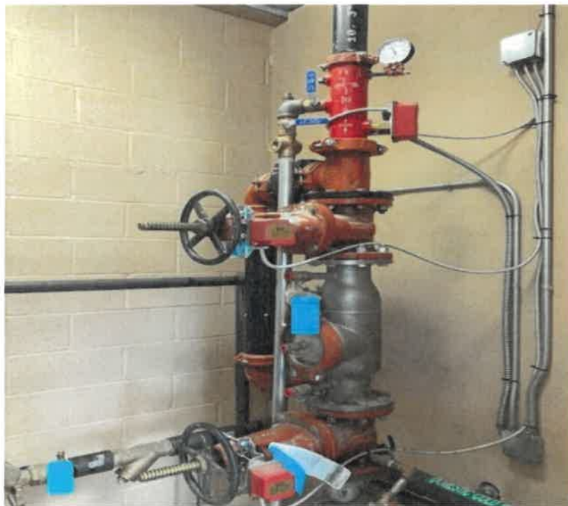
Utility room in Pool hallway.
