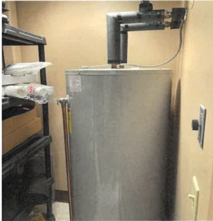
Hot water heater located in Maintenance/Utility closet.
