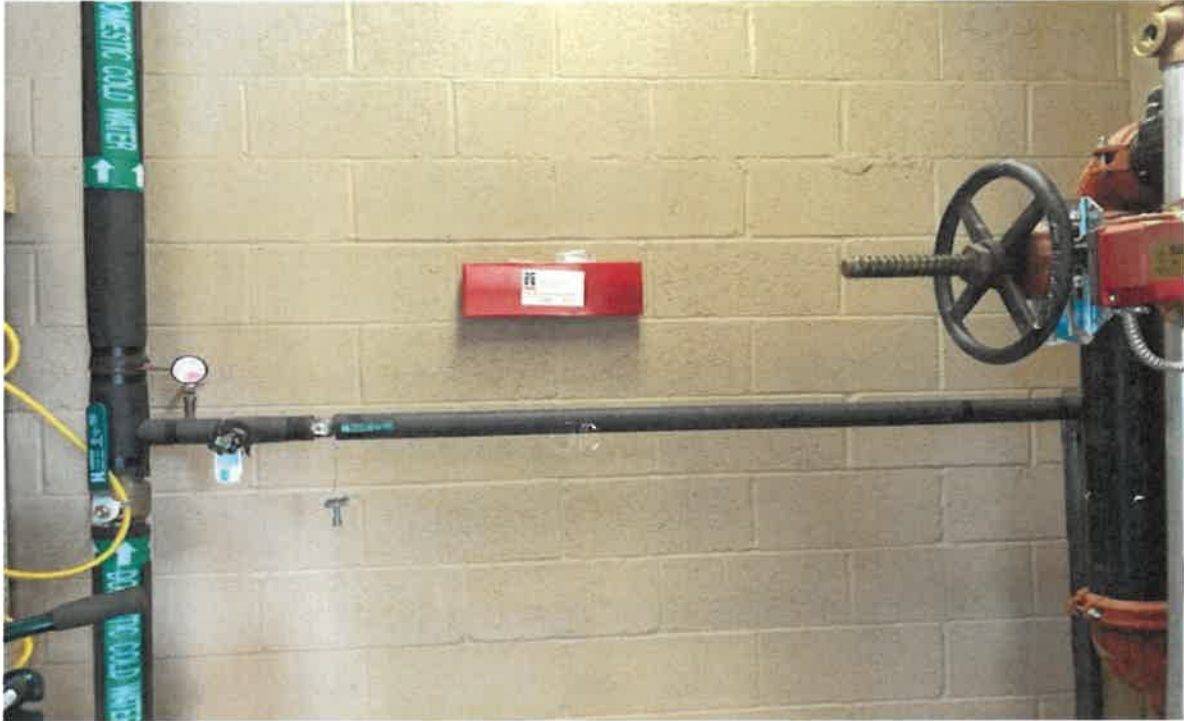
Utility room in Pool hallway.
