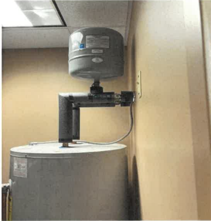
Maintenance/Utility closet viewing the hot water heater
